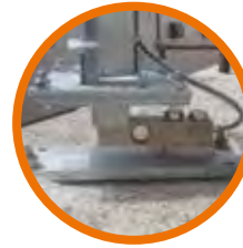
Silo Loadcell Weighing System
